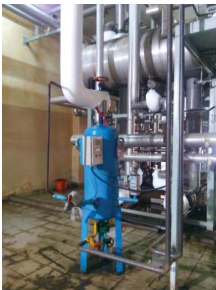
Figure 2: Ammonia Dehydrator Installation
